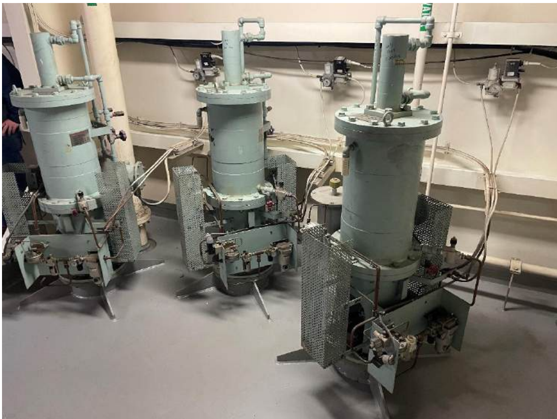
Photo 46 – Typical condition of valve actuators on the starboard safety deck
