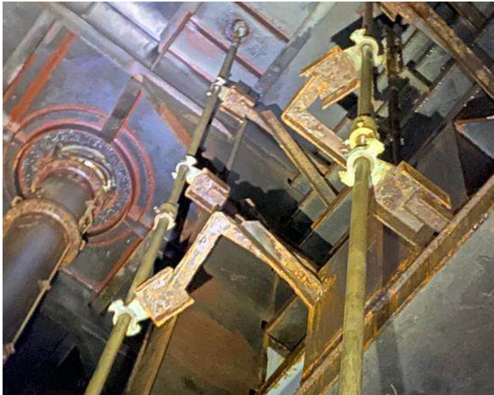
Photo 68 - Tank 1 AFT - S: Angled Reach Rod Guides
