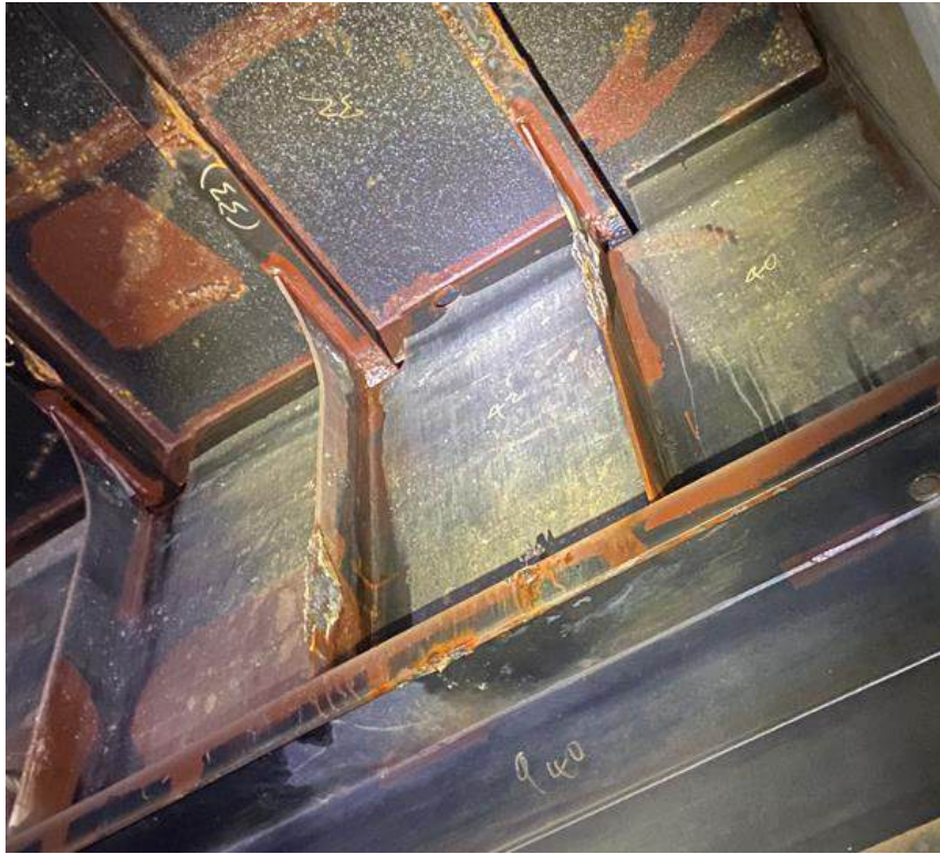
Photo 100 - Tank 6 AFT- P (Fr 10, 12, 13): OVHD FBs on OCL WT BHD Notching/Scaling
