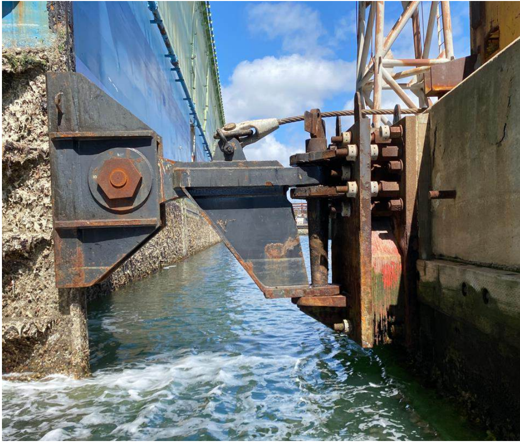
Photo 39 - Condition of Frame 121 Gripper
