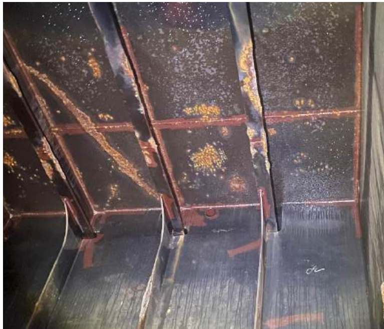
Photo 82 – Tank 4-P (FR 92): Pontoon deck stiffener notching 4-ft form off-CL longitudinal WT BHD. Others have rust scale in this bay.
