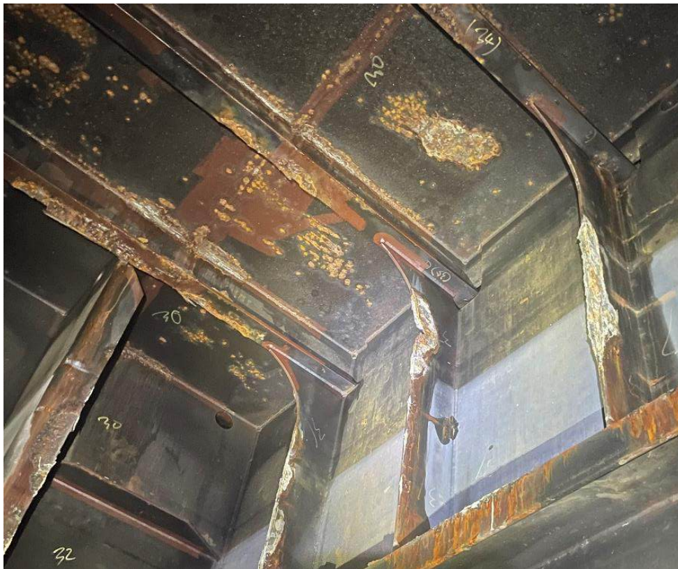
Photo 60 – Tank 1 AFT-P (FR 204): Vertical flat bar at the top of the off-CL longitudinal WT BHD is notched. Adjacent pontoon deck stiffeners in this area have rust scale
