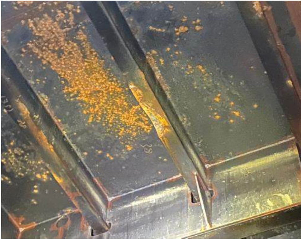
Photo 71 - Tank 2 FWD – P (Fr 204): PD Stiffener in Bay 2 Iso Flg Notch
