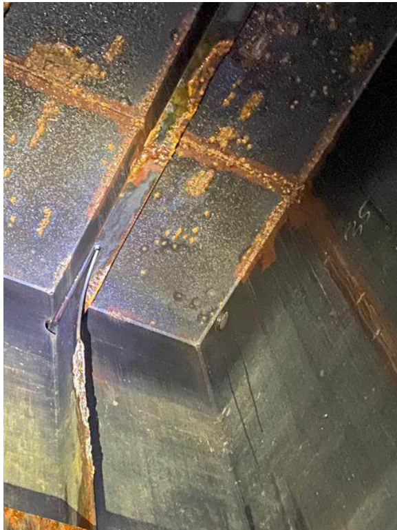
Photo 72 - Tank 2 FWD - P (Fr 185): FB on OCL WT BHD Notch/Scale, PD Stiffeners Similar
