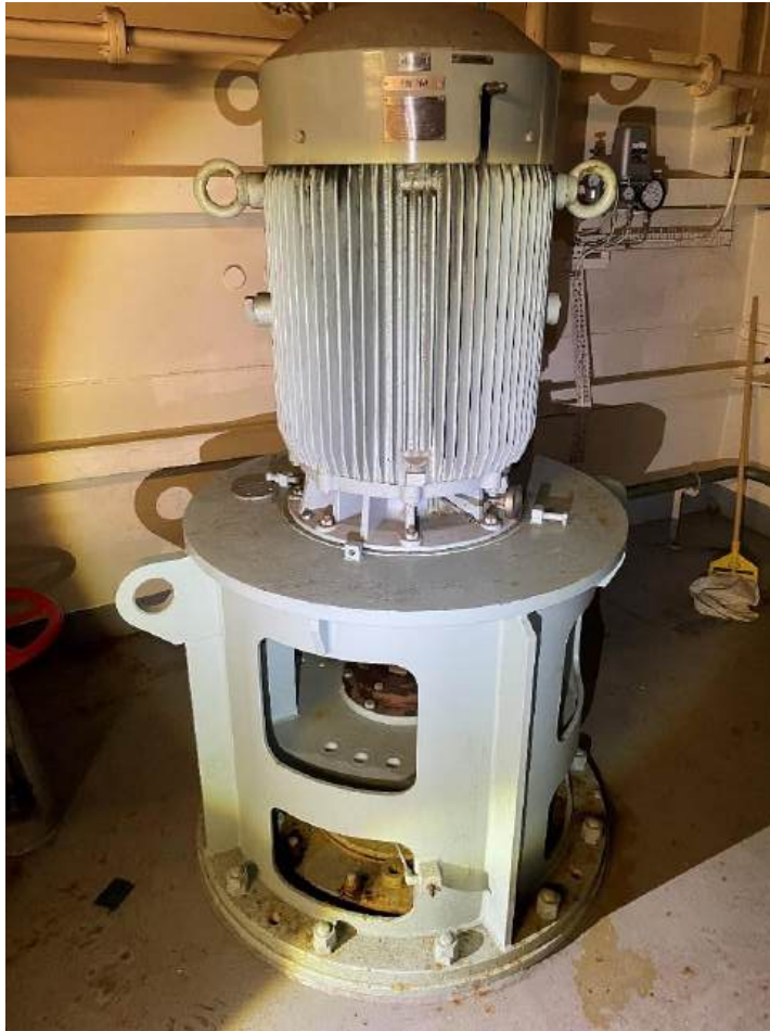
Photo 47 – Typical condition of fire pump (Port shown)
