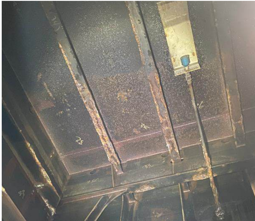
Photo 56 - Tank 1 FWD – PC: PD Stiffeners KE & Neck
