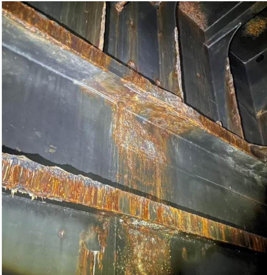
Photo 85 – Tank 5S (FR 41): On the off-CL longitudinal WT BHD, stiffeners 4 & 5 are scaling.
