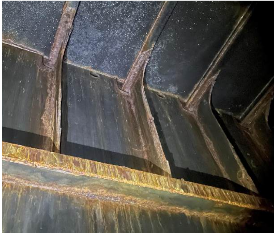
Photo 86 – Tank 5A - S (FR 41 (63, 64)): On the off-CL longitudinal WT BHD, the vertical flat bars have MRS with connection to pontoon deck stiffeners
