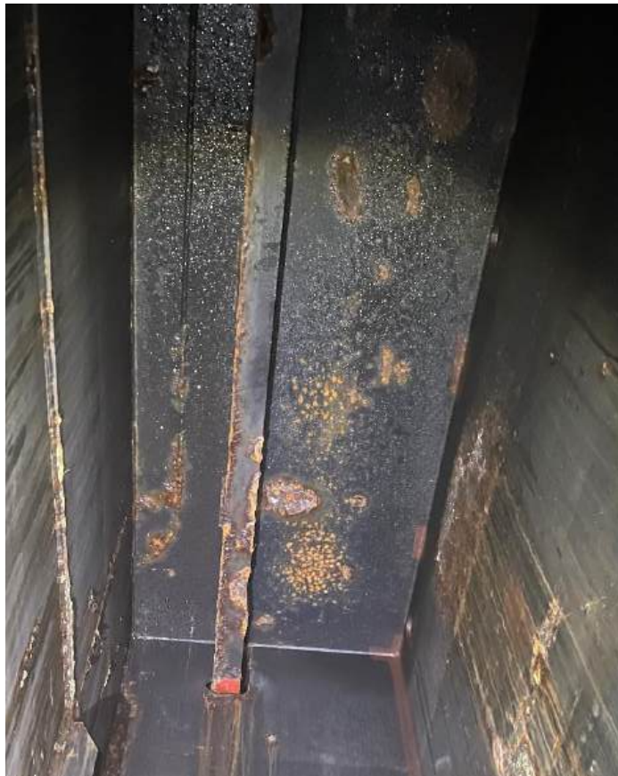
Photo 66 – Tank 1 AFT-SC (FR 222): Pontoon deck stiffener notching near off-CL longitudinal WT BHD
