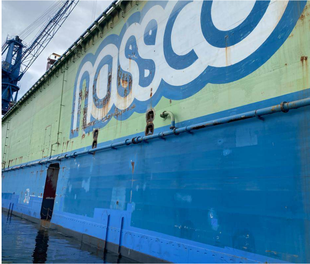
Photo 27 - Typical Condition of OTBD Shell (STBD)
