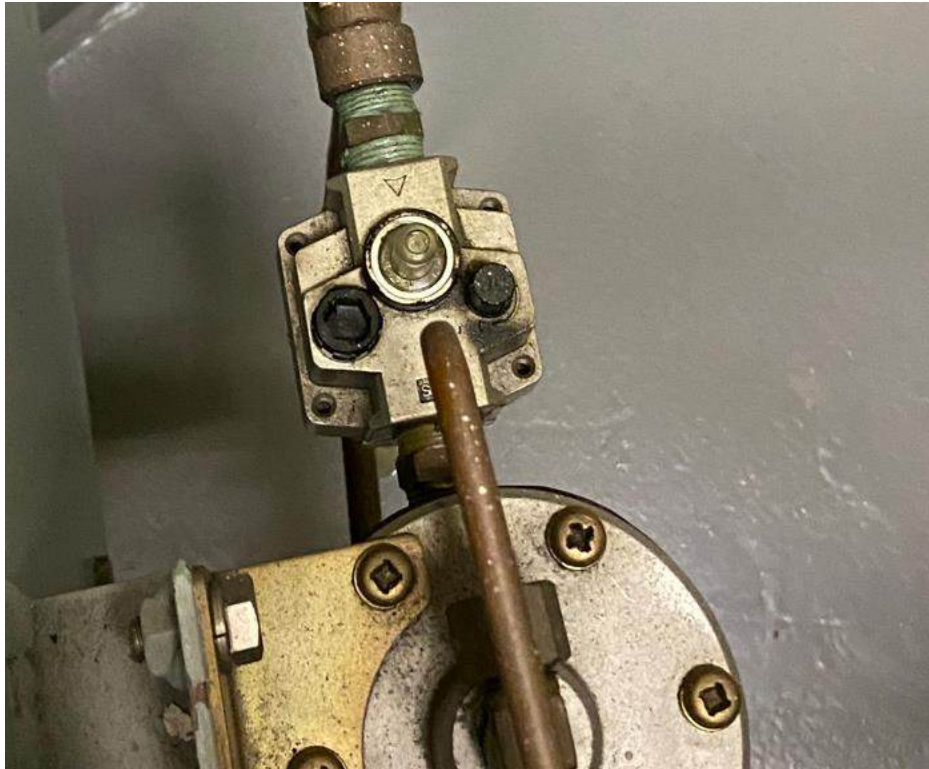
Photo 52 - Missing Cap on Air Line Filter
