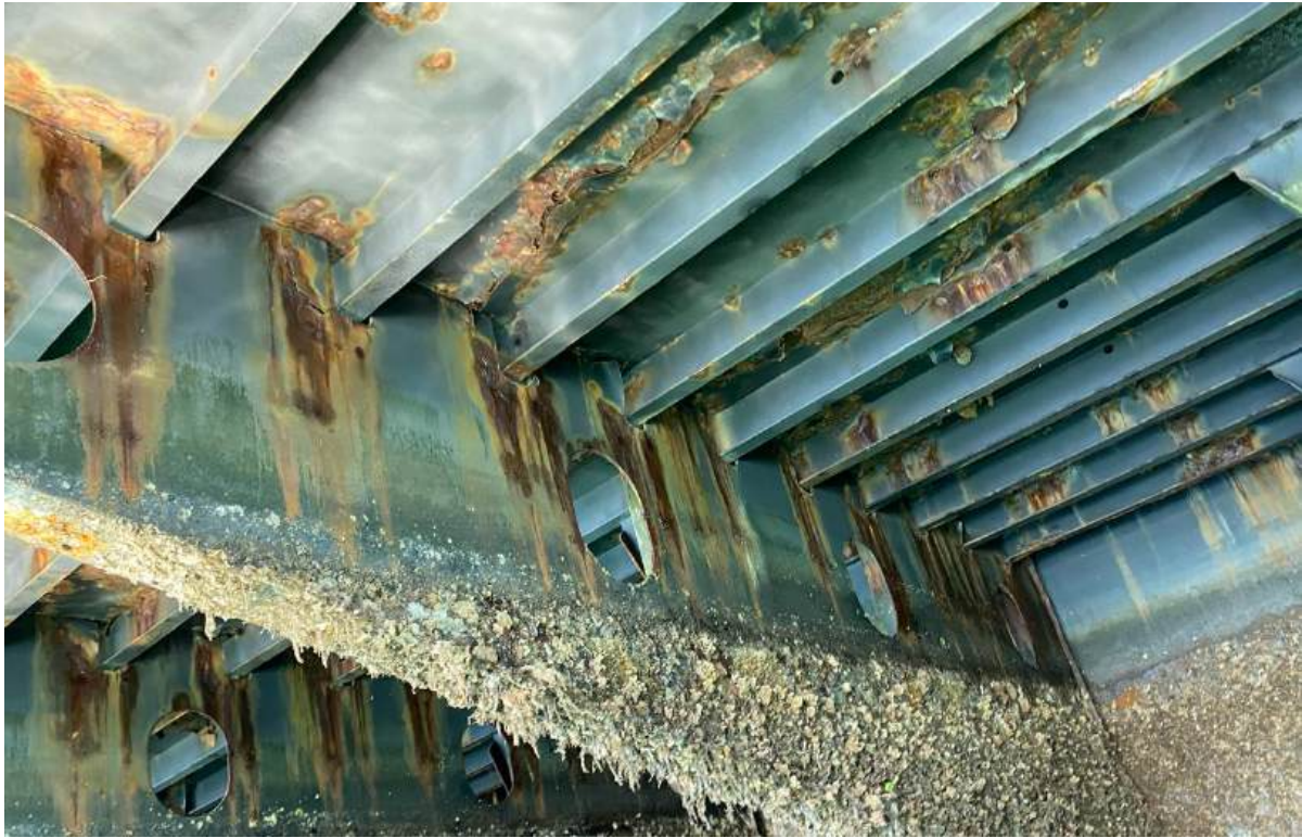
Photo 33 - Condition on Underside of Apron
