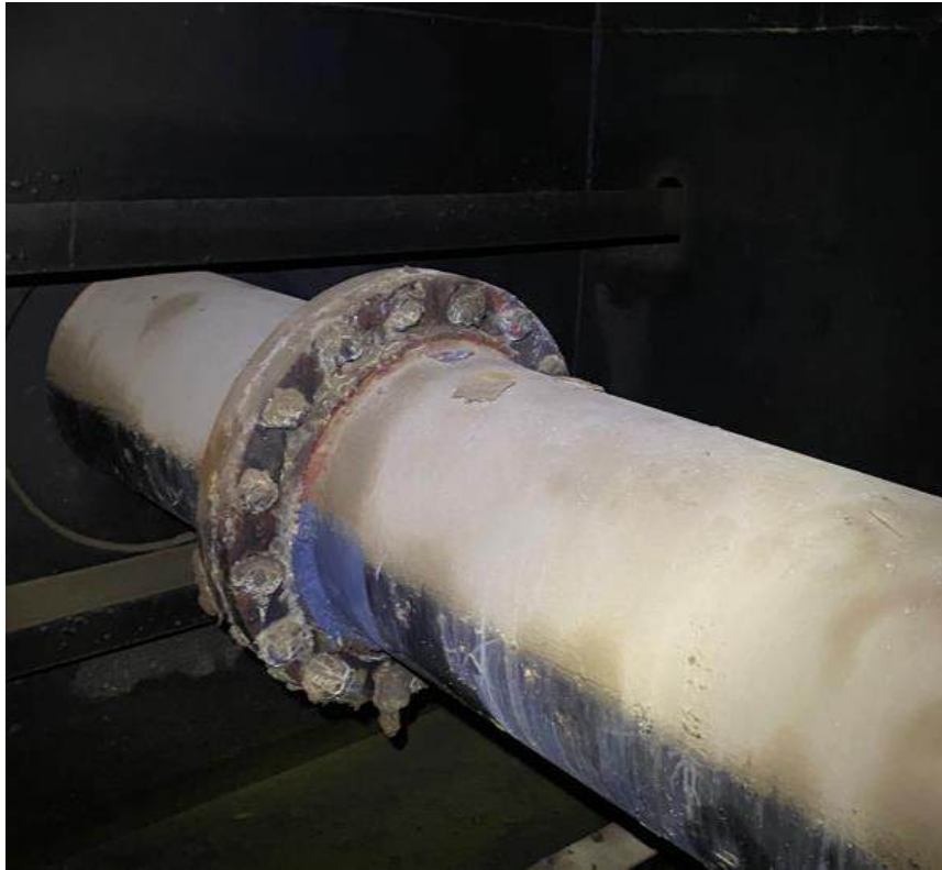
Photo 7 - Typical Condition of Ballast Flanged Connection
