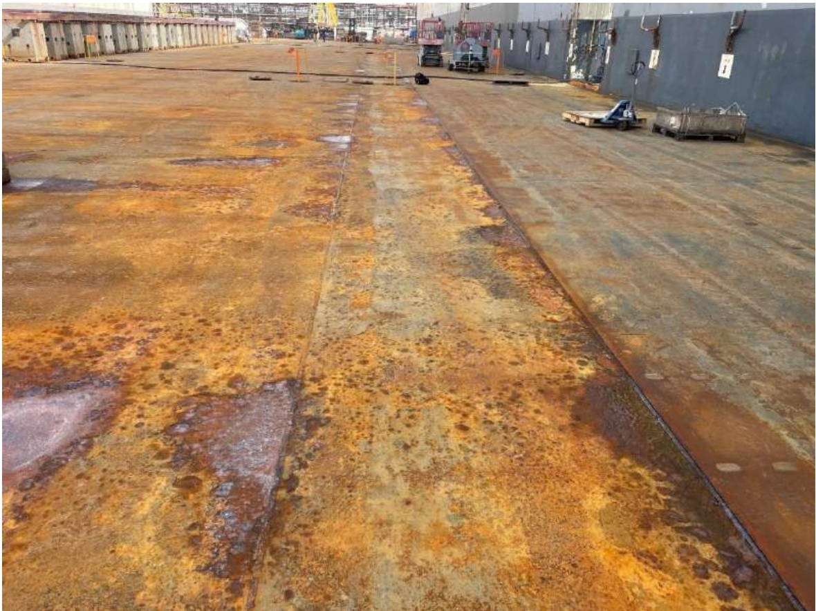
Photo 20 – Typical condition of the pontoon deck
