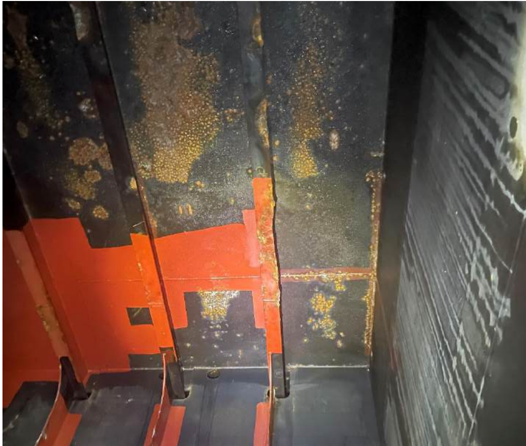
Photo 61 – Tank 1 AFT-P (FR 207): Pontoon deck stiffener notched midspan between off-CL BHD and 1st longitudinal OTBD
