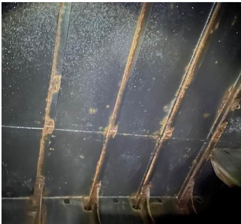
Photo 87 – Tank 5A - S (FR 41 (50-55)): Pontoon deck stiffeners in this bay have MRS on the flanges
