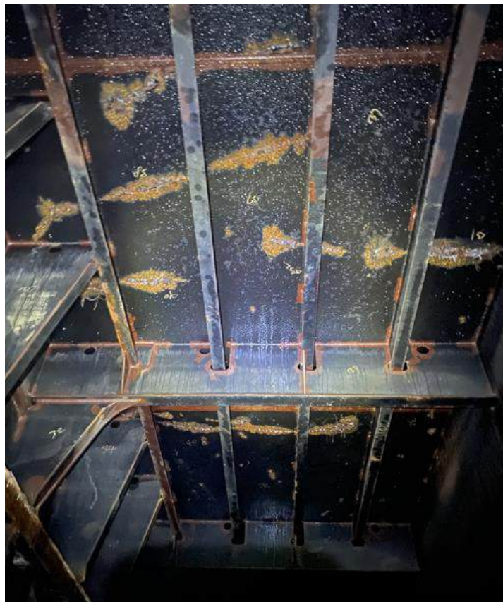
Photo 12 - Condition of Underside of Pontoon Deck
