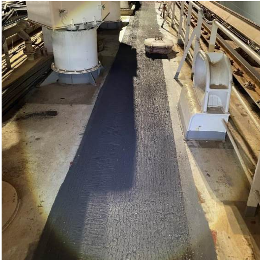
Photo 23 – Condition of STBD Wing Deck
