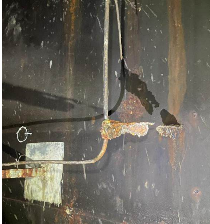
Photo 84 – Tank 5S (FR 45): Piping Sensor has wasted support bracket
