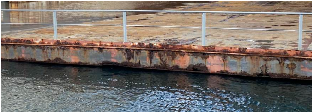
Photo 32 - Condition of Apron Coaming
