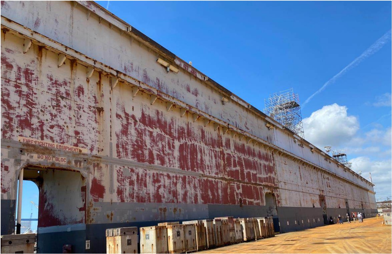
Photo 29 - Typical Condition STBD INBD Wing Shell
