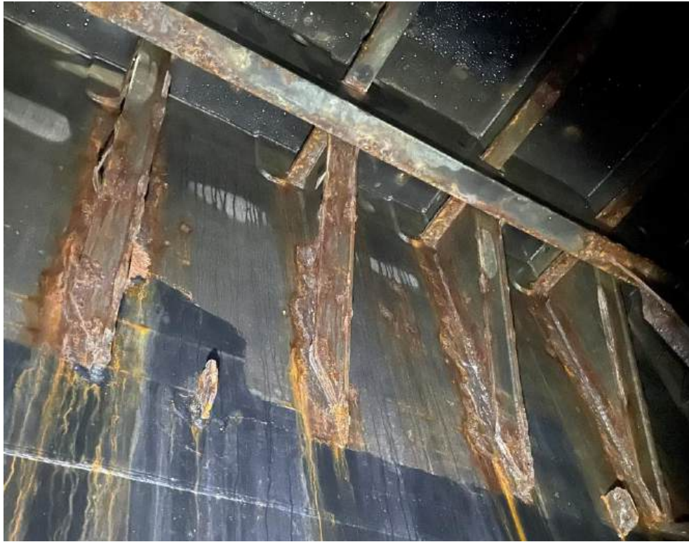
Photo 98 – Tank 6 FWD-SC (FR 36-41): Scaling of CL BHD and connection to transverse PD stiffener brackets
