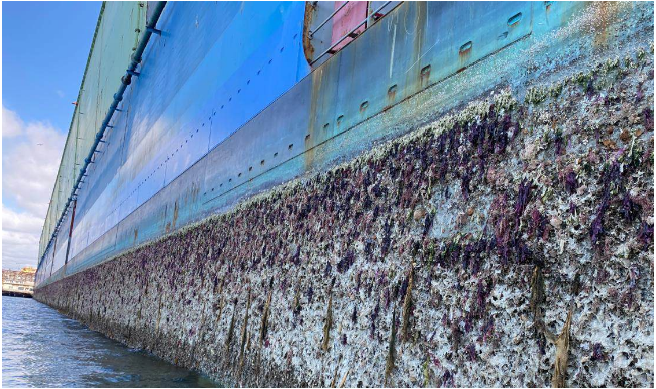
Photo 25 - Pontoon Shell Typical Condition
