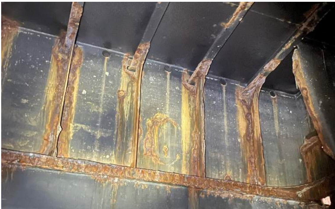
Photo 91 – Tank 5B AFT-S (FR 41(5-10)): On the off-CL longitudinal WT BHD, the upper vertical flat bars have M-HRS along with their adjacent pontoon deck stiffeners
