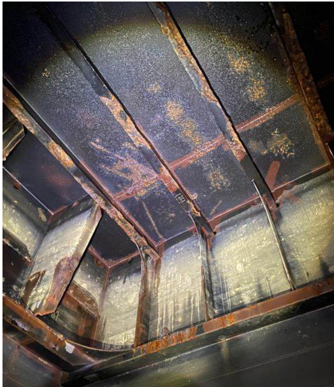
Photo 101 - Tank 6 AFT- P (Fr 12, 14, 15): PD Stiffeners in Bay 1 Flanges Notched
