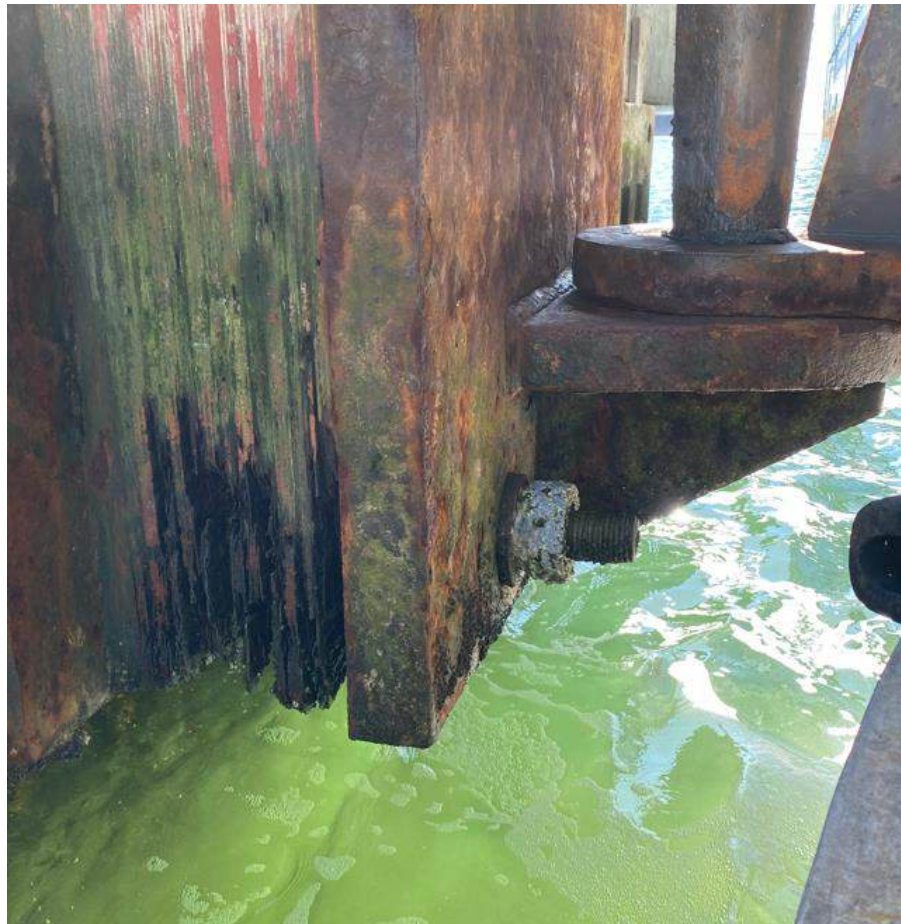
Photo 41 - Condition of Lower Anchor Bolt, Nut, and Timber Frame 121
