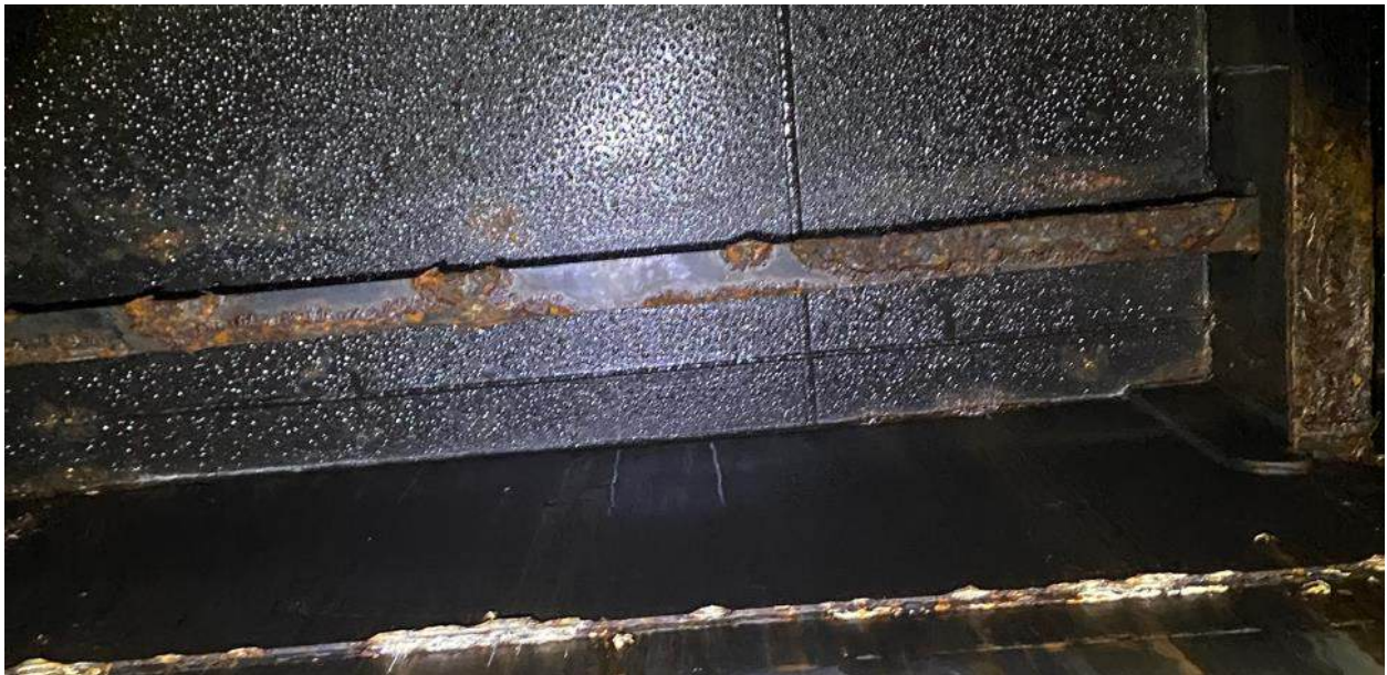
Photo 64 - Tank 1 AFT - PC (Fr 222): PD Stiffener KE and Notch Iso Areas (x12)
