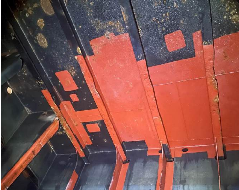
Photo 63 – Tank 1 AFT-P (FR 219-220): These pontoon deck stiffeners are notching from the off-CL longitudinal WT BHD to the 1st longitudinal OTBD.
