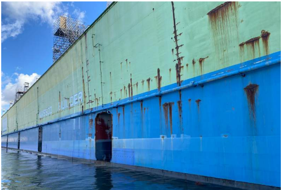
Photo 28 - Typical Condition of OTBD Shell (Port)
