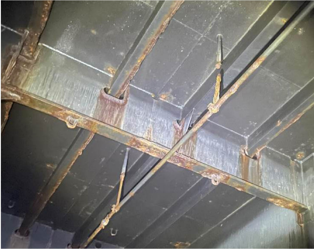
Photo 55 – Typical abandoned overhead piping with wasted hangers
