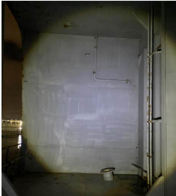
Photo 54 - Lack of Vent Pipe Extension
