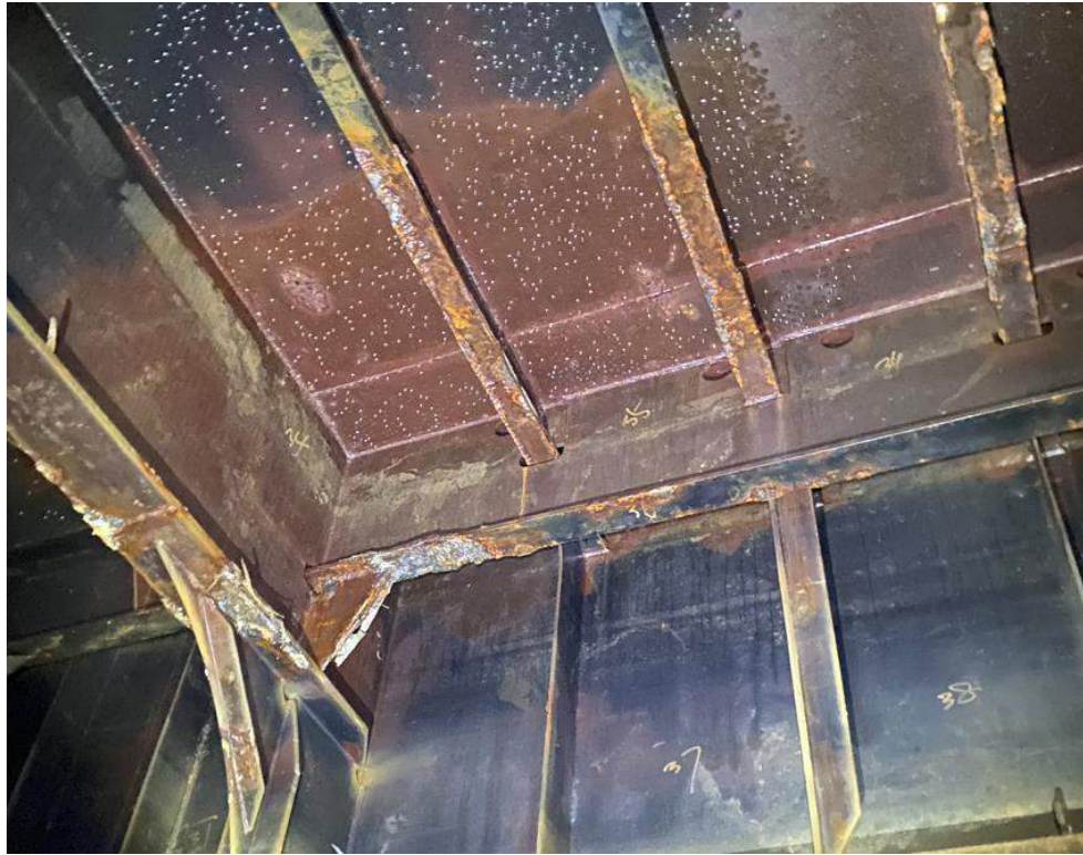
Photo 57 - Tank 1 FWD – PC: PD Stiffeners KE & Neck
