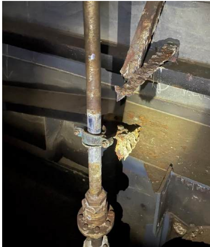
Photo 81 – Tank 3-S (FR 151): Wasted lower reach rod support to flood valve
