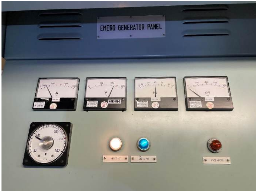
Photo 48 – Emergency generator panel (Powering 2 ballast pumps)
