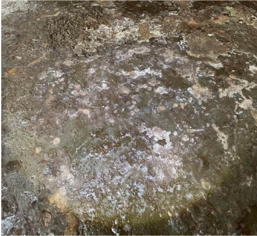
Photo 21 – Scaling and Pitting of the pontoon deck plate
