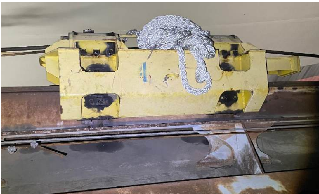
Photo 42 – Typical condition of vessel handling trolley
