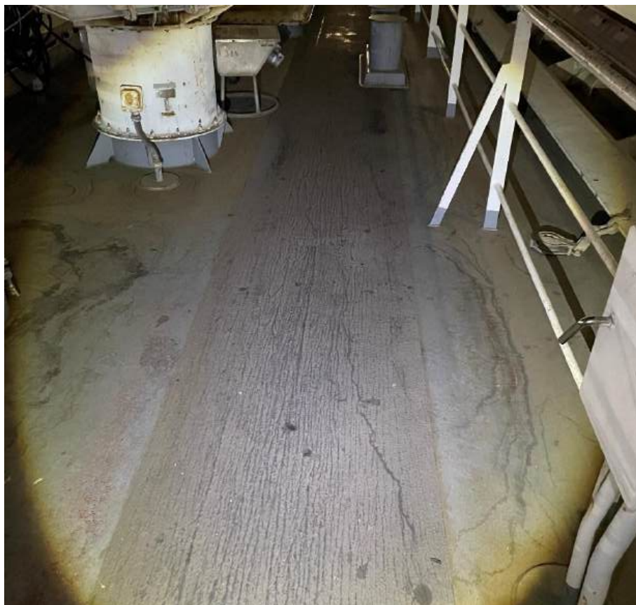
Photo 24 – Condition of PORT Wing Deck
