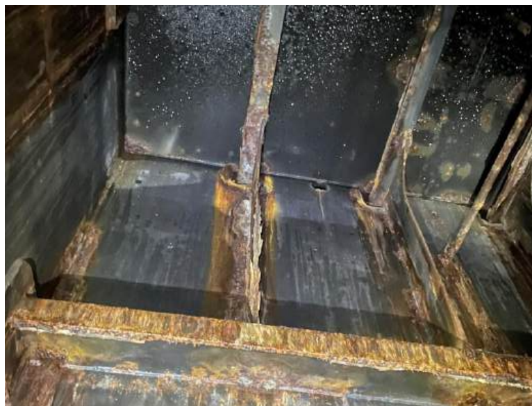
Photo 89 – Tank 5B FWD-S (FR 41(30-35)): On the off-CL longitudinal WT BHD, the upper vertical flat bars have M-HRS along with their adjacent pontoon deck stiffeners
