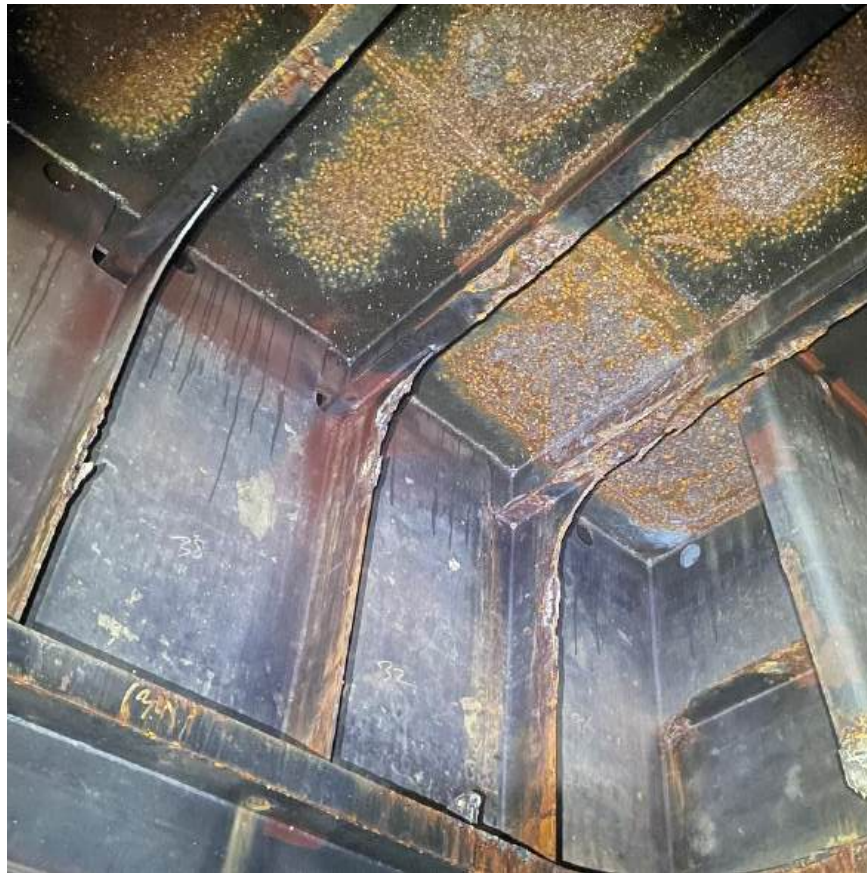
Photo 79 – Tank 2 AFT-S (FR 173-174): Pontoon deck stiffeners and flat bars have HRS/moderate notching at the off-CL longitudinal WT BHD
