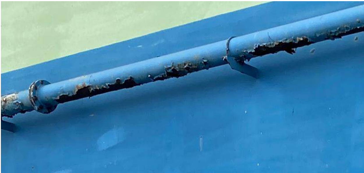
Photo 51 - Exterior Fire Main Pipe
